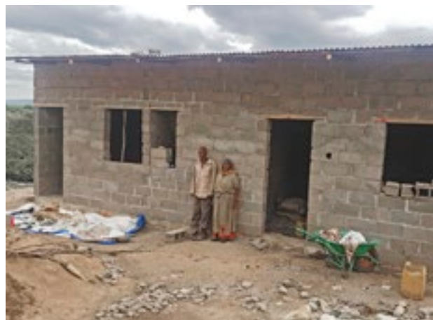
Nine houses and sanitary facilities for families in need are constructed in Ethiopia with the financial support of the foundation.
